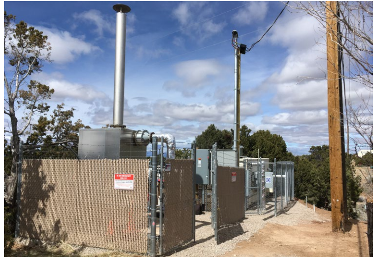
DBS&A creatively engineered larger SVE equipment to fit within a space that is shared by highway ROW and a utility corridor.
