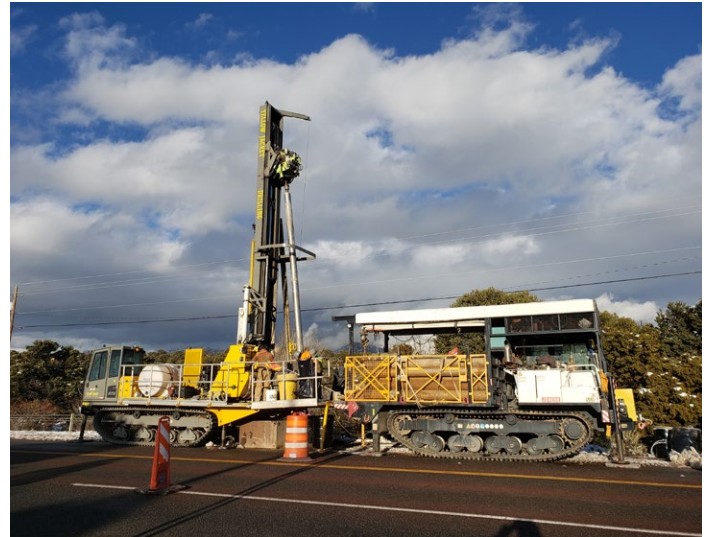
DBS&A provided oversight and CQA for the installation of 20 wells, most of which were installed in highway ROW.
