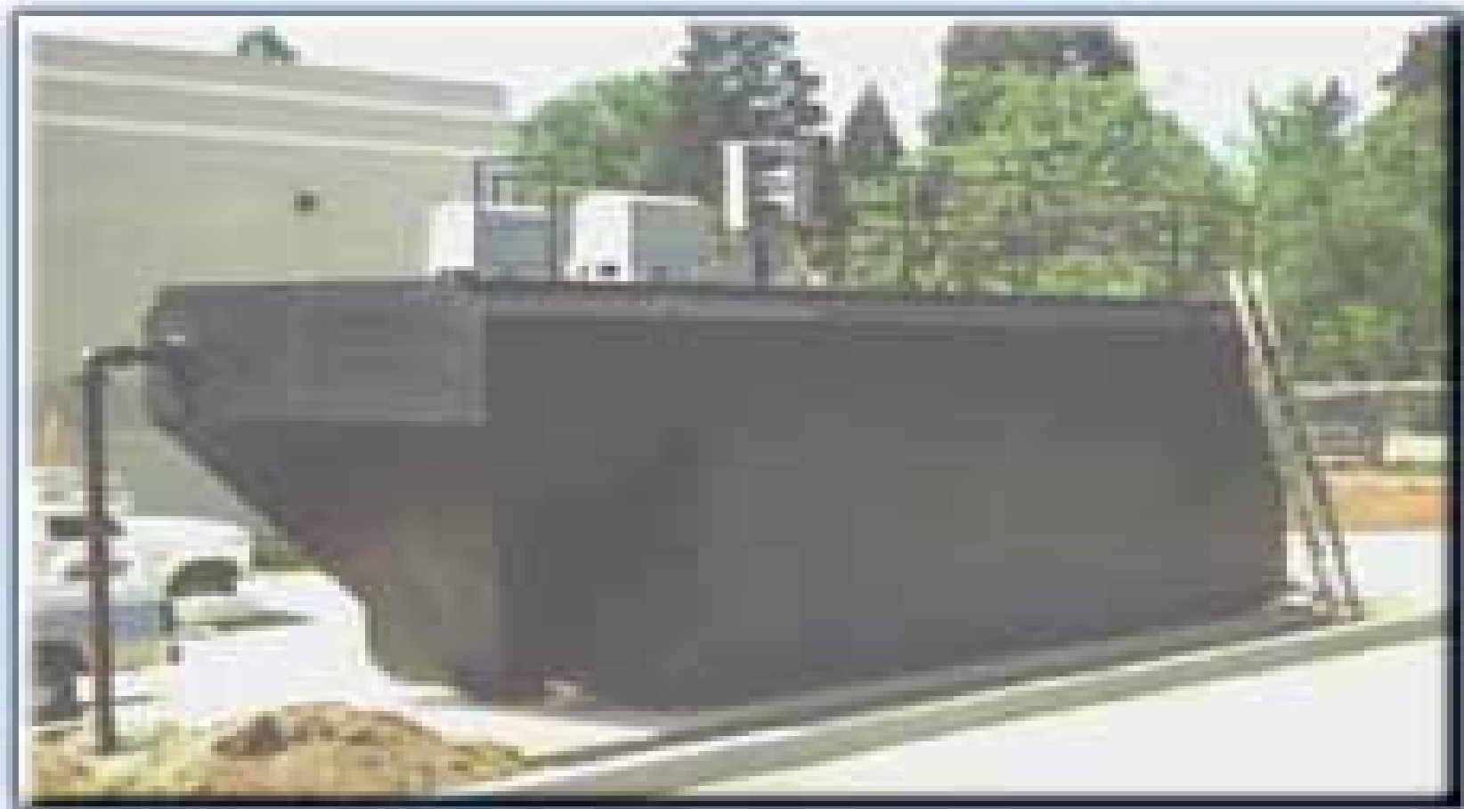
PACKAGE TREATMENT PLANT
