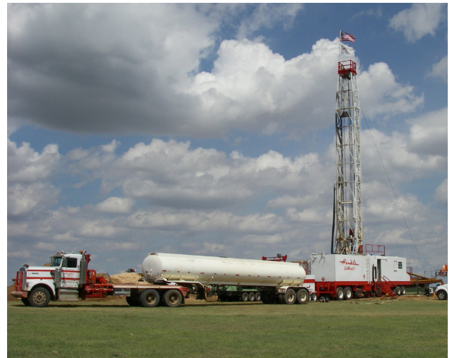
Optimal sites for the initial prototype well installations were based on a 3D hydrostratigraphic model.
